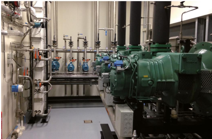
Industrial heat pump at Hutten slaughterhouse
