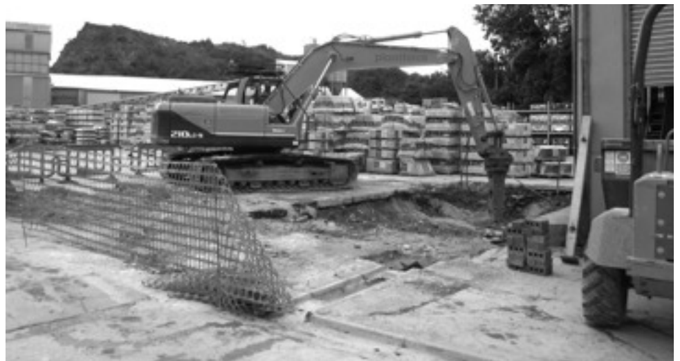
Excavation of the new settlement tank near the quarry entrance in August 2012
