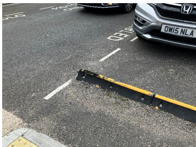
Figure 28 – Poor pavement condition along The Beach
