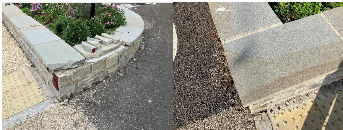
Figure 27 – Damaged planter next to the mini roundabout
