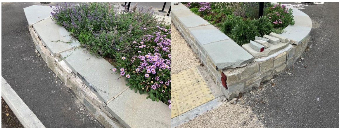
Figure 26 – Damaged planter at the corner of junction The Beach/ Elton Road
